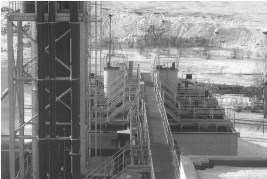
Fig. 6. View of the HDS plant at Ronneburg (2-train / 4-step neutralization and de-carbonization tower on the left-hand side)
